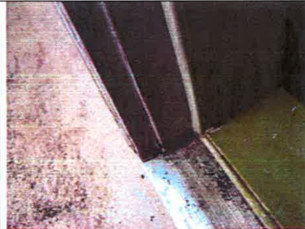
Photo 18: Unit 306 - Deteriorated wood frame of the swing door
