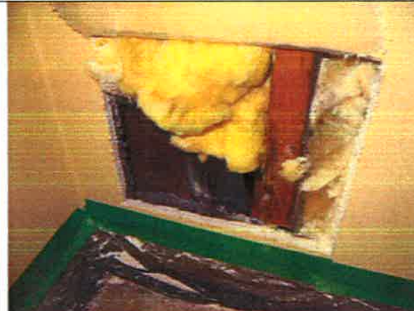
Photo 16: Unit 108 - Interior exploratory opening to review the drain in the exterior wall
