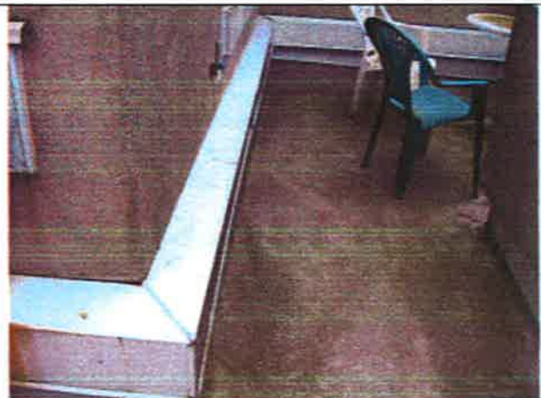
Photo 22: Amenity Unit - Vinyl deck membrane with staining
