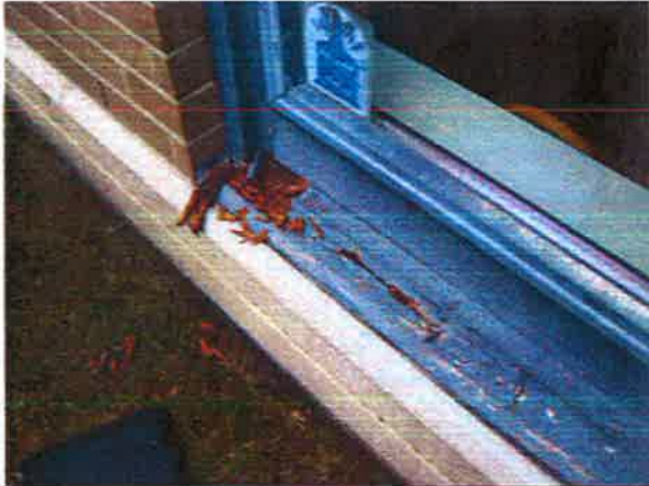
Photo 13: Deteriorated wood condition at the window sill of the brick veneer cladding
