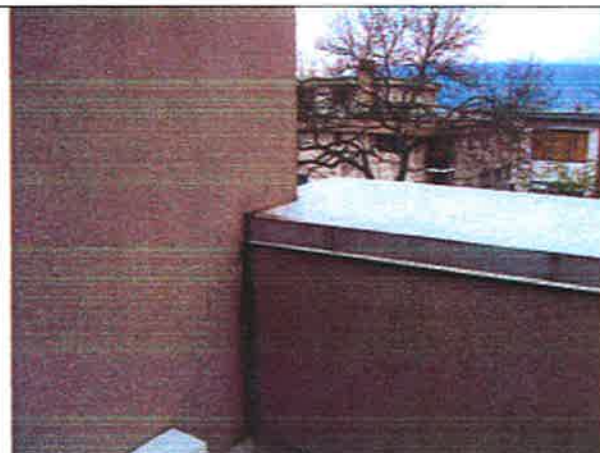
Photo 23: Amenity unit – Extensive staining of the parapet cladding at saddle and exploratory opening from earlier investigation
