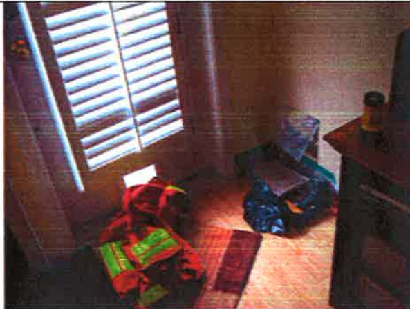
Photo 15: Unit 108 - Interior exploratory opening to review the drain in the exterior wall
