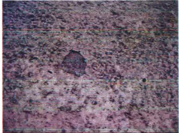
Photo 20: Unit 306 – Cracked and delaminated balcony deck membrane
