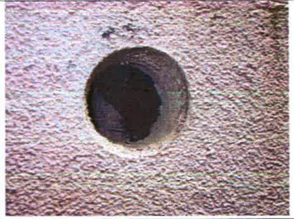
Photo 10: Exploratory Opening at the EIFS below window sill in the east elevation
