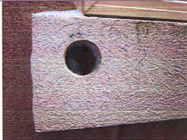
Photo 9: Exploratory Opening at the EIFS below window sill in the east elevation
