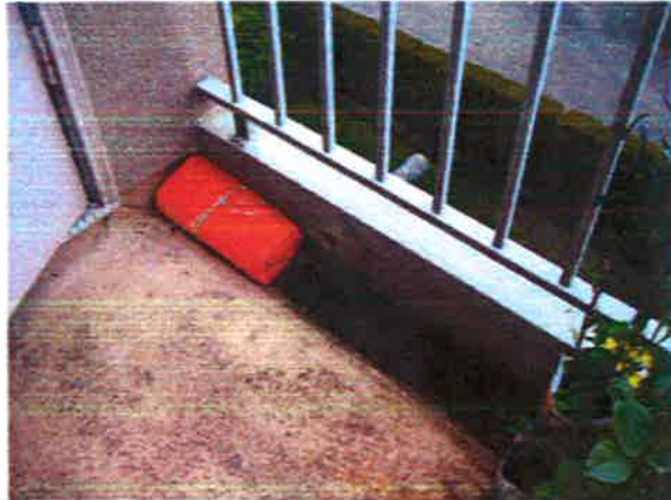
Photo 19: Unit 306 – Extensive staining at the tough of the balcony deck
