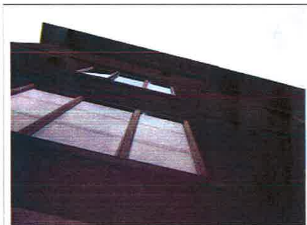
Photo 1: Unit 206 – Appears a localized rehabilitation of the exterior wall and window was conducted
