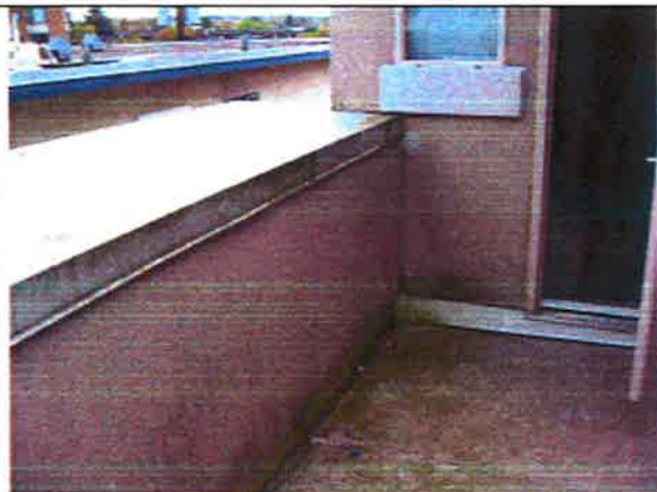
Photo 21: Amenity Unit - Vinyl deck membrane with staining
