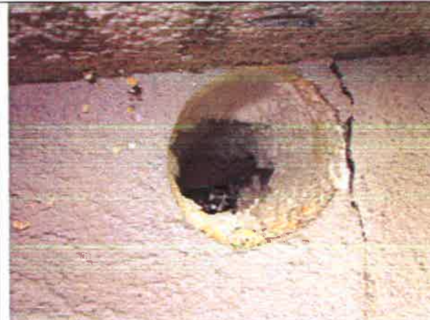
Photo 12: Exploratory opening adjacent to the crack in the EIFS band
