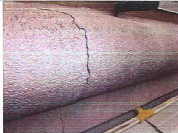
Photo 11: Crack in the EIFS band
