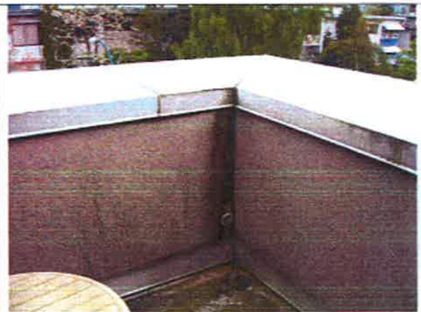
Photo 24: Amenity Unit – Extensive staining of the parapet cladding at saddle and exploratory opening from earlier investigation
