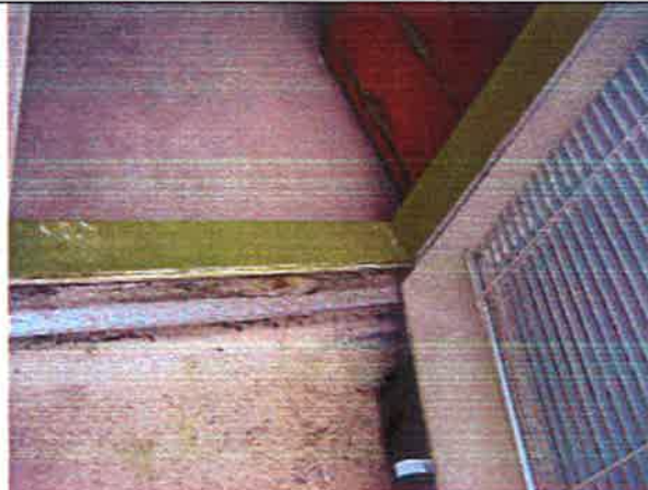
Photo 17: Unit 306 - Evidence of water ingress and deteriorated wood frame of the swing door
